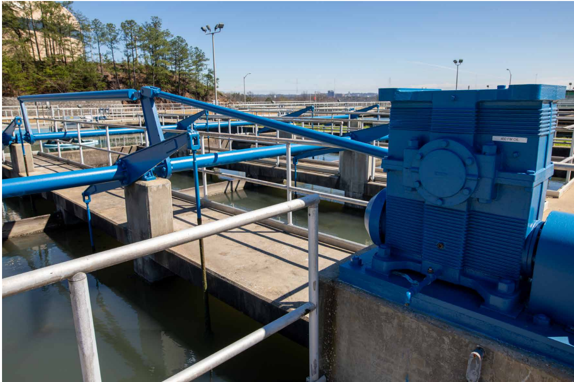
WESTERN FILTER PLANT
