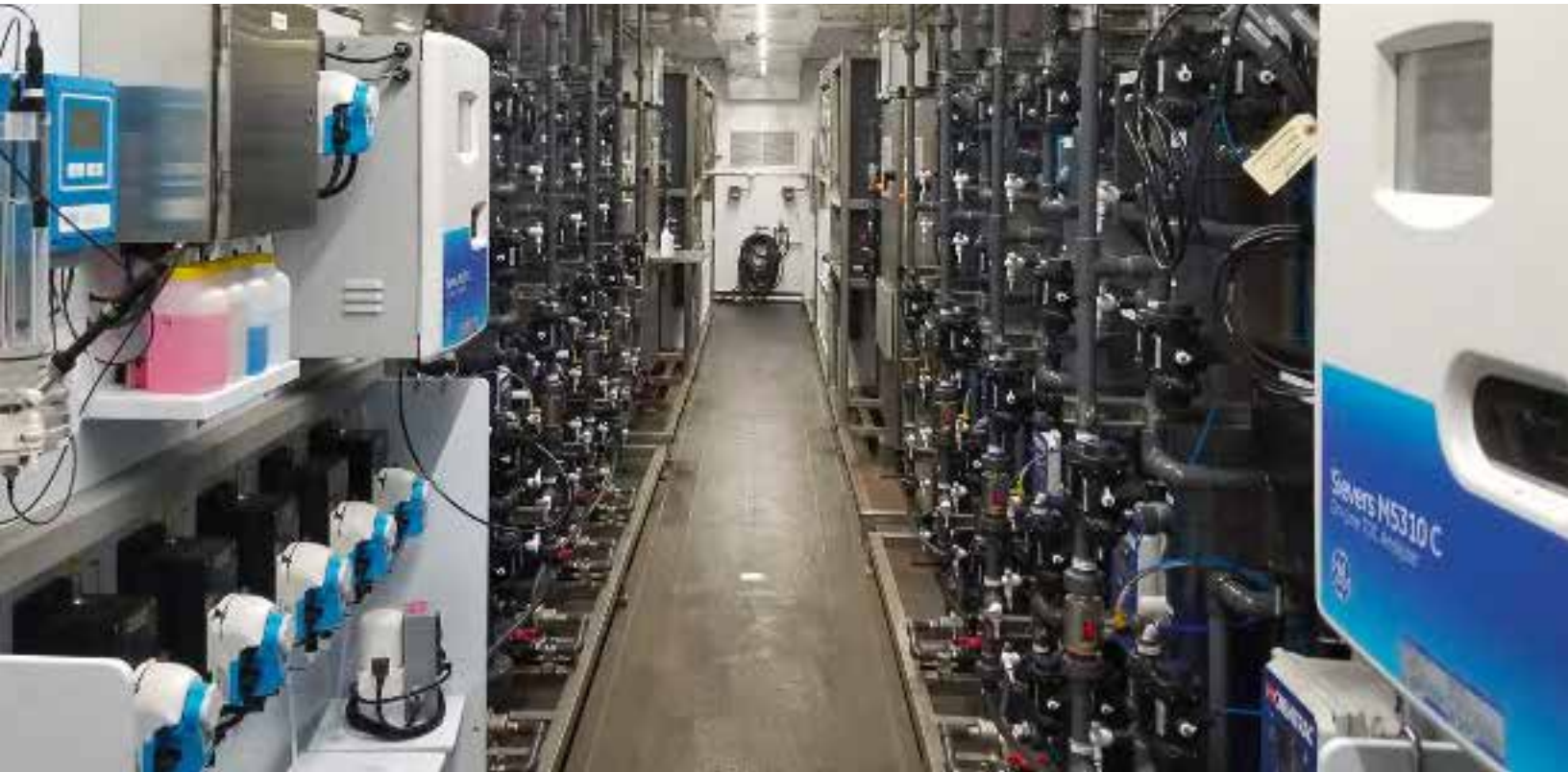
BWW'S MOBILE PILOT PLANT TESTS WATER PROCESS TREATMENT ALTERNATIVES.
